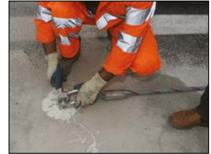
Figure 17 - Cables connecting to front pickets
