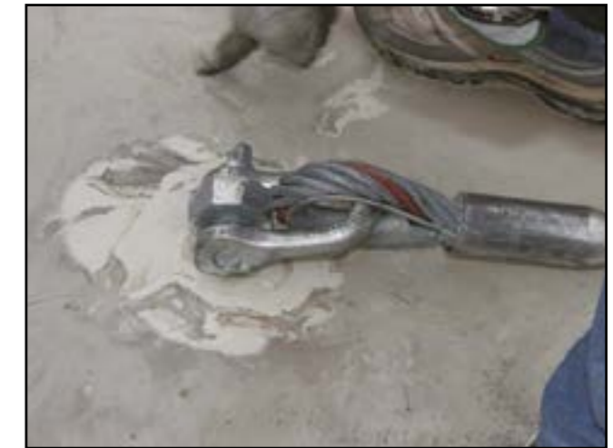
Figure 18 - Cables connecting to front pickets
